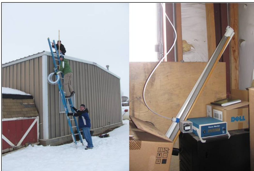
Figure 3-1. Installation of the sample line and 2B Ozone Monitor at the Roosevelt location.
